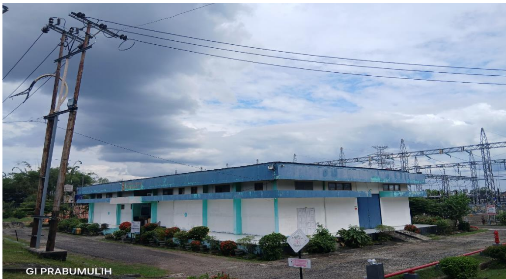
Figure 1. Operational Building at the Prabumulih Substation.
